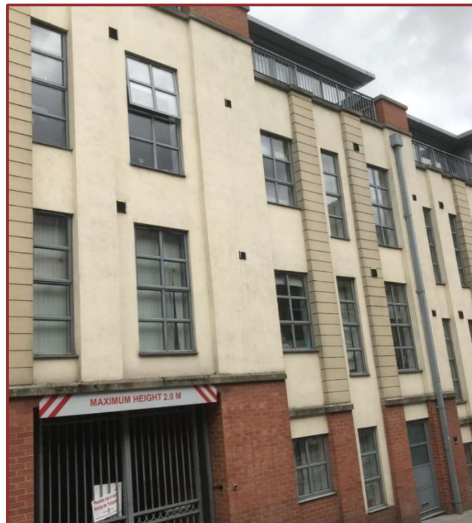
South facing elevations to Castle Exchange consisting of glazing, masonry and render
